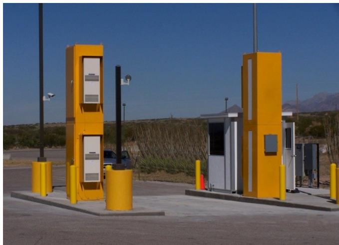
Figure 2 Installed HPGe Portal at Anthony, New Mexico
