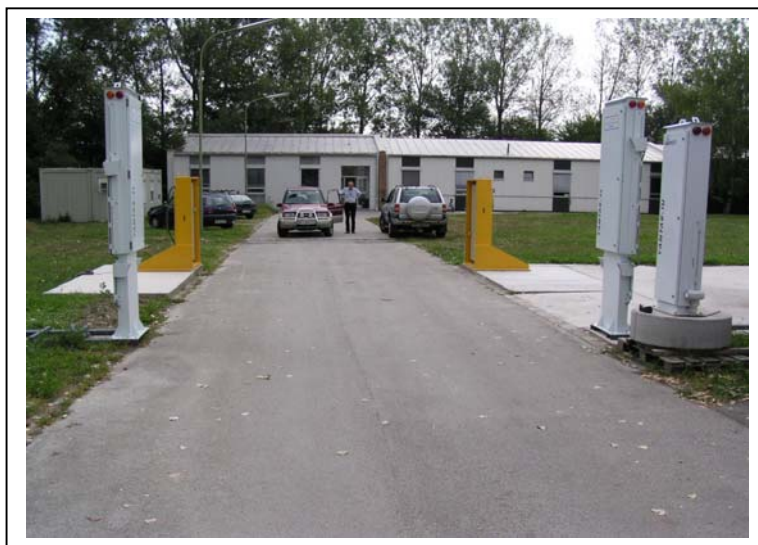
Fig. 8: AT900 system (yellow pillars near the cars) installed at the ITRAP laboratory test site
